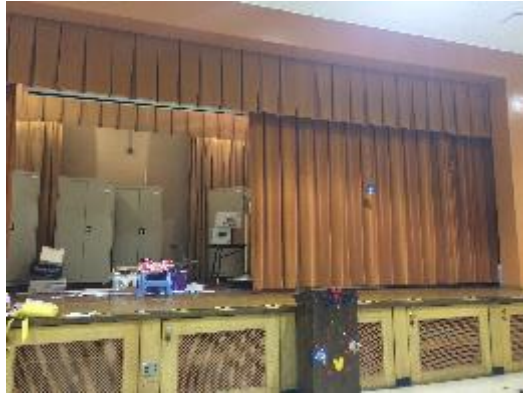
Dated worn out finishes
