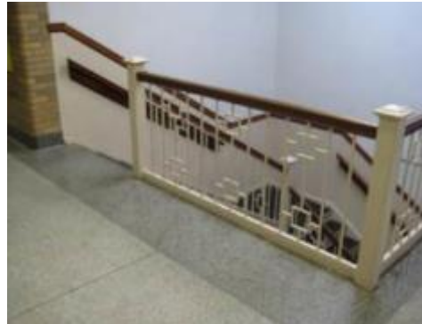
Non-Code compliant hand/guardrails
