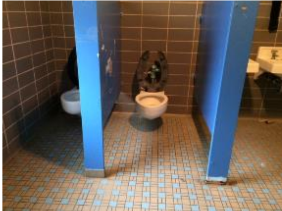
General finishes and fixtures worn
