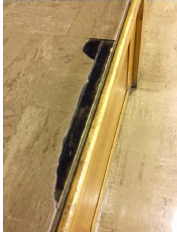
Damaged VAT (asbestos flooring)
