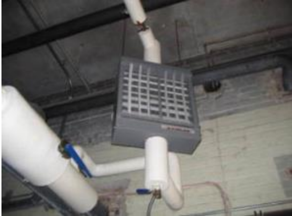
Heating water unit heater
