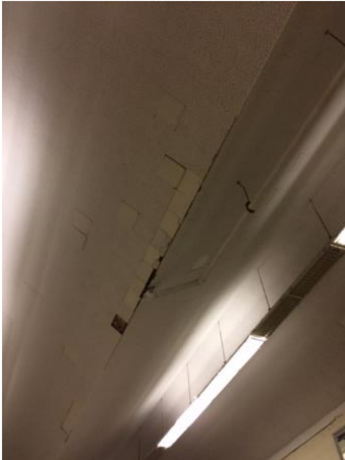
Gym roof tiles deteriorating from roof leaks
