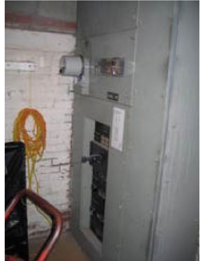
Main Electrical Distribution panel – system cannot be expanded to accommodate A/C
