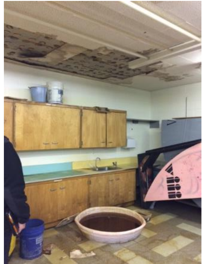
Significant Roof leaks and damage
